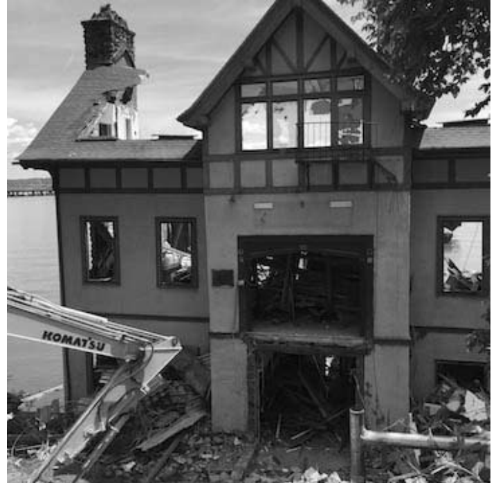
The old Grand View village hall is demolished, another victim of Superstorm Sandy. Vince O'Brien photo
