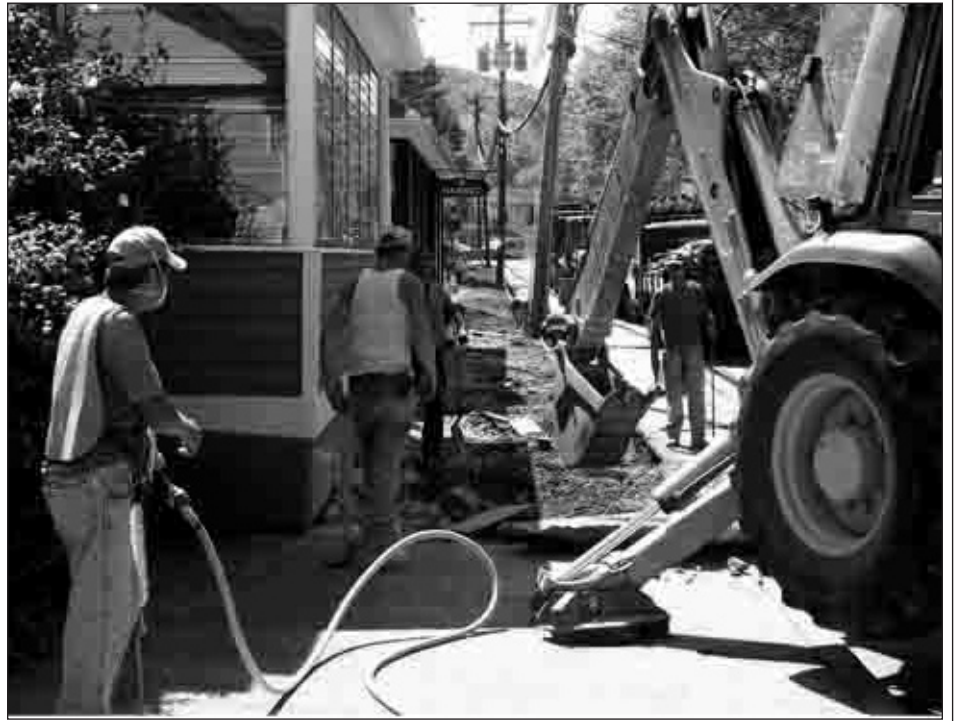
Dig they must for a better Piermont: sidewalk reconstruction on Main Street. Photo by Fred Burrell.
