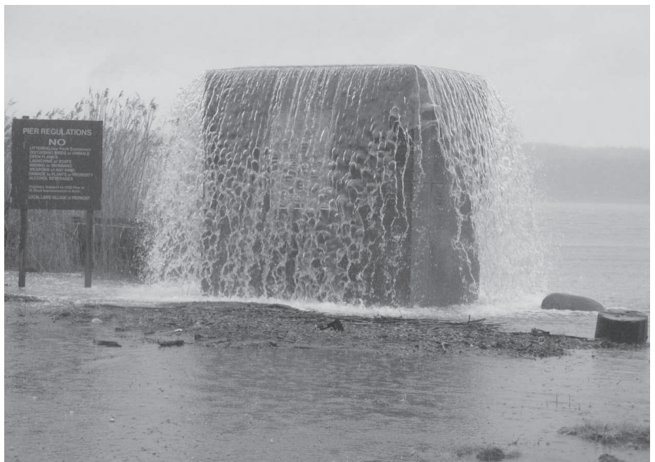
Overflow gushes from sewer outflow connection box on Pier Road during heavy rain. Photo by Margaret Grace
